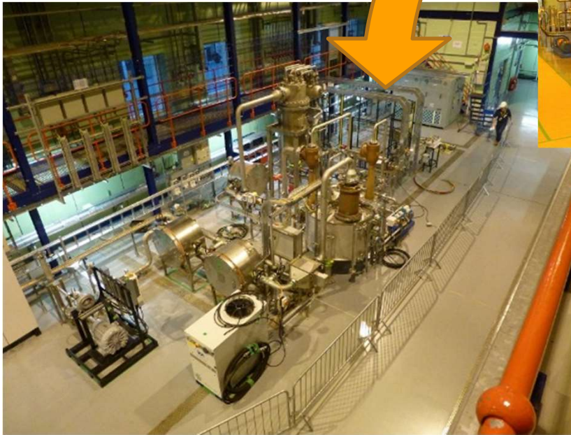
Off-Gas Treatment System
