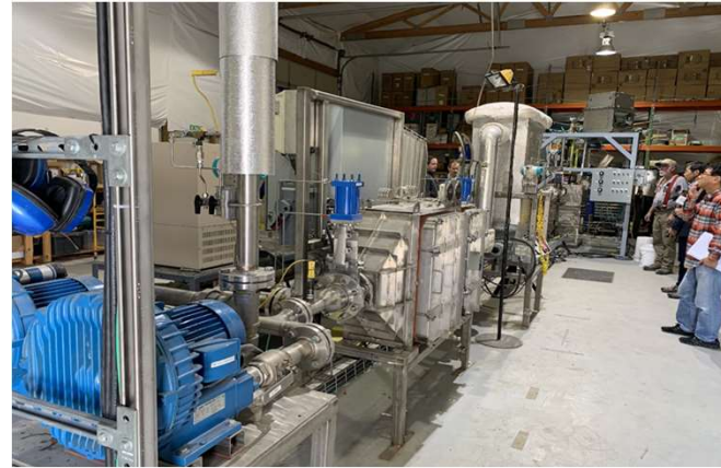
Off-Gas Treatment System
